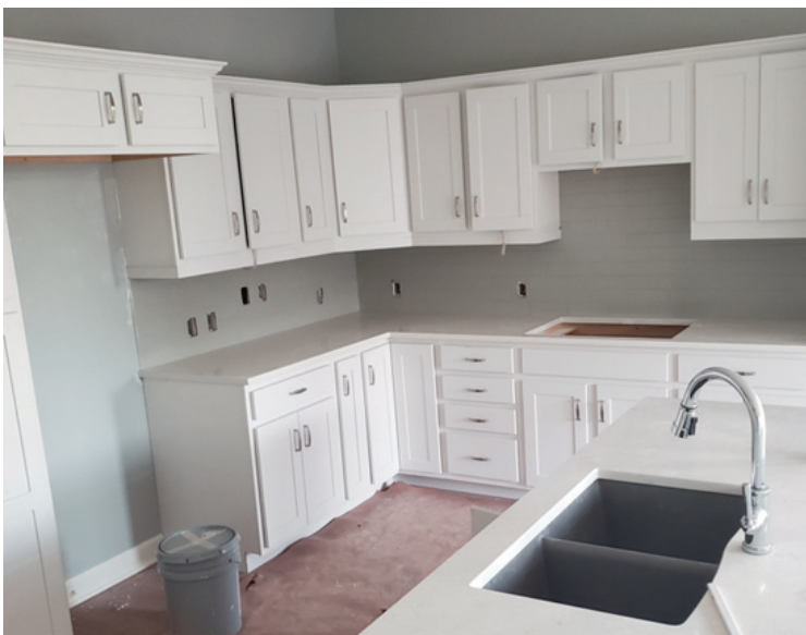
The interior of the new Meadows East Expansion is really taking shape as crews are completing cabinetry installation including in the kitchens and bathrooms. Interior painting is also progressing nicely.
